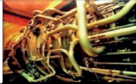
GUPCO Turbines – Ras Shokier, Egypt
